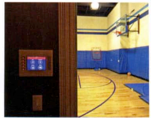
The audio system functions as an intercom for the house, and all touchscreens are equipped with mics and speakers. The page ability extends to the basketball court located under the garage on the lower level.
